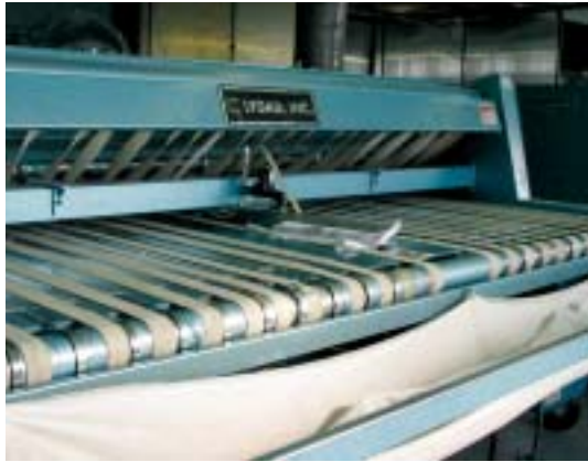
A flatwork ironer in the plant
