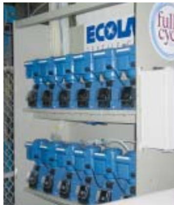
A look at the plant's chemical injection equipment
