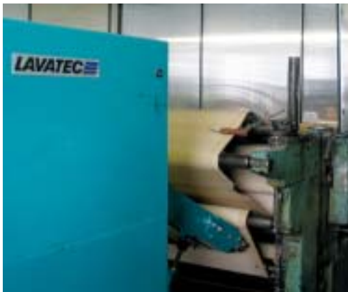
Another view of the plant's flatwork finishing equipment
